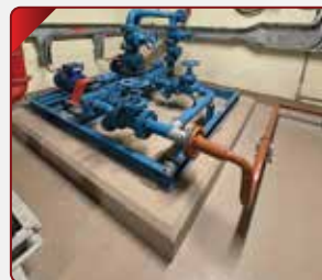
Plumbing & Domestic Water
